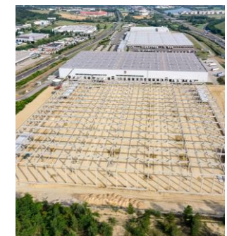
ctPark Budapest W. (199k sqm) Adjacent to M0 and M1 motorway and train tracks between central Budapest and Komárom (city on Danube river)
